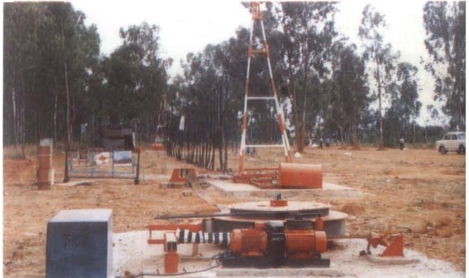
Aircraft arrester barrier system
