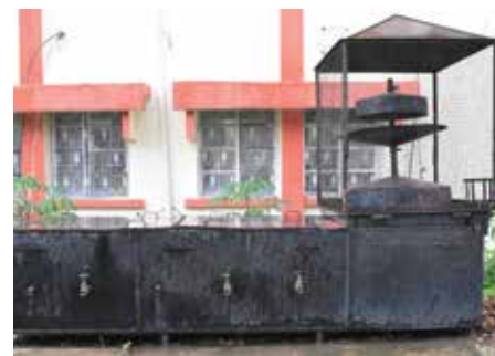
Iron Removal Unit (3000l/hr)
