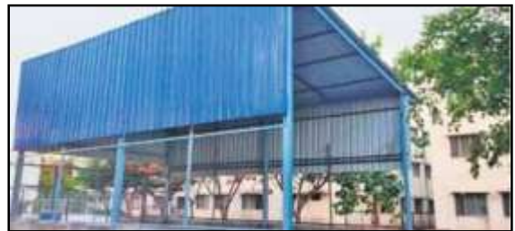
The structure for DRDO's proposed medical oxygen plant at Koppal Institute of Medical Sciences in Karnataka
