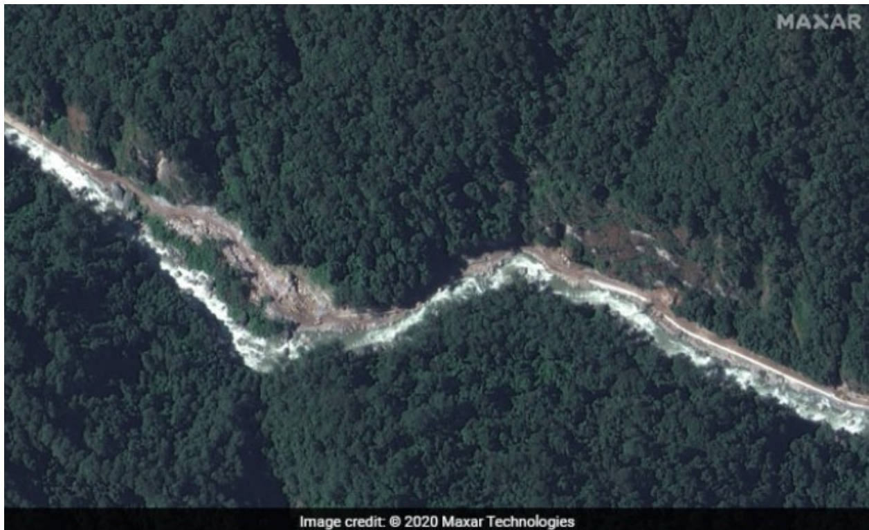
Road construction along Torsa river, Bhutan. Copyright: Maxar Technologies 2020. Click here for high resolution image
