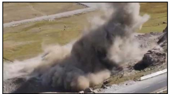
Work began on the Zoji La tunnel near Drass on Thursday with Union Minister Nitin Gadkari initiating the first blast for the project.(HT PHOTO)
