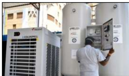
The DRDO recently installed high capacity medical oxygen plants at AIIMS Trauma Centre for Covid-19 patients.(ANI Photo)
