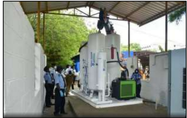
A Pressure Swing Adsorption oxygen plant being installed at Tiruchi Mahatma Gandhi Memorial Government Hospital. | Photo Credit: M. Srinath
