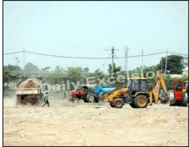
Men and machinery at work near Amarnath Yatri Niwas, Bhagwati Nagar in Jammu where DRDO is setting up a 500-bed hospital.— Excelsior/Rakesh
