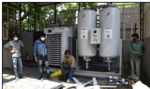
Final touches being made to the DRDO's oxygen plant at RML hospital, Delhi | Sanjay Ahlawat
