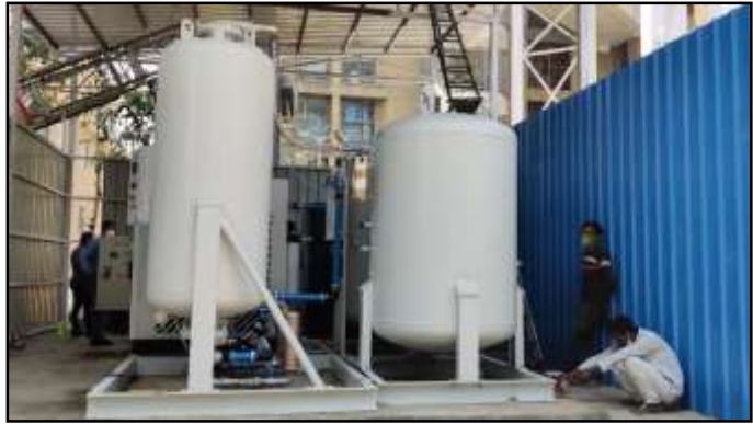
The DRDO will be installing five such plants in Delhi to help hospitals meet their demands for medical oxygen.
