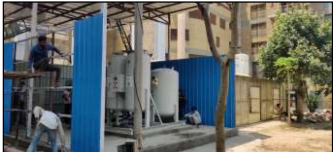
The oxygen plant installed by the DRDO at AIIMS New Delhi.
