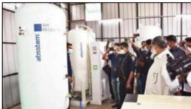
An oxygen plant is set to become operational at Ambala civil hospital
