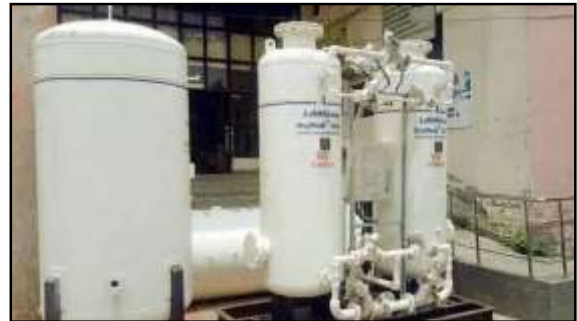
An oxygen plant with a capacity of 1,000 LPM (litres per minute) is being installed at the ESI Hospital and will cost ₹1.7 crore. This oxygen plant, which is nearing completion, has been funded by HITES (HLL Infra Tech Services Ltd) under the ministry of health and family welfare (HT Photo)
