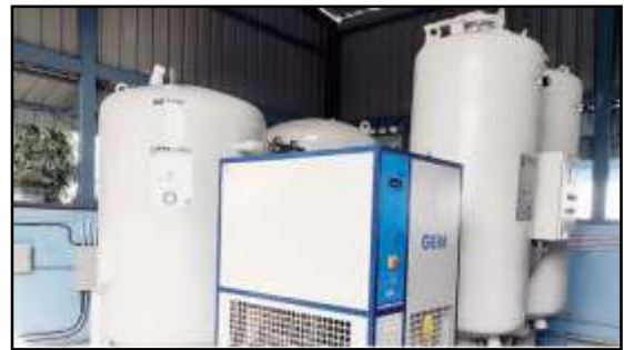
A view of the machinery at the oxygen plant inaugurated at the NBMCH, on the outskirts of Siliguri. (Passang Yolmo)
