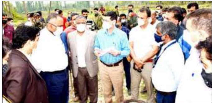
Div Com taking stock of ongoing construction work of DRDO 500 bedded Covid hospital.
