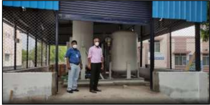
A new oxygen generator is under installation in Virudhunagar Government Medical College Hospital in Virudhunagar on June 05, 2021. | Photo Credit: The Hindu
