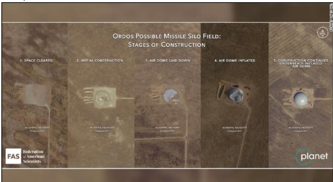
Different stages of construction underway by Chinese engineers on multiple silos at the possible Ordos missile silo field in August 2021. After clearing the space for the project, they use inflatable domes to protect the active construction on the silos.
