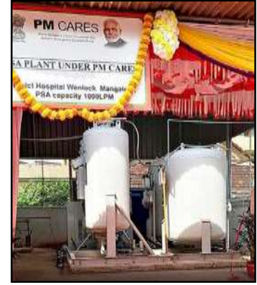
The 1,000 litres per minute capacity oxygen generation plant that was formally commissioned at the Government Wenlock Hospital in Mangaluru on Thursday.
