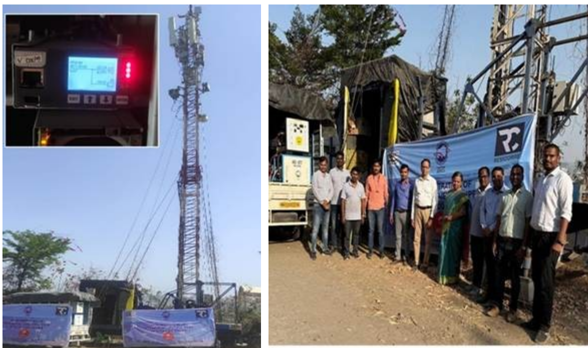
Figure: (Left) Telecom tower powered by mobile PEM Fuel Cell unit with the inset showing the current rating drawn from Fuel Cell at the Base Transceiver Station. (Right): The Fuel cell system along with the demonstration team.
