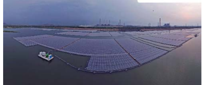
At Ramagundam, the solar modules are placed across 500 acres on floaters manufactured with high-density polyethene material that keeps floating irrespective of water-level fluctuations.
