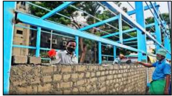
Construction of medical oxygen generator plants progressing at the Government Mohan Kumaramangalam Medical College Hospital in Salem on Tuesday.
