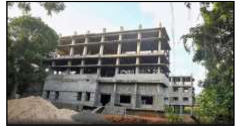
The building being constructed for research and testing in food, pharma and genetics on Andhra University campus in Visakhapatnam on Saturday. | Photo Credit: K.R. Deepak
