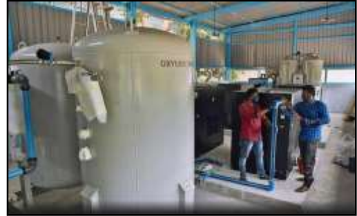
Works under way to set up oxygen generator plant at the Government Mohan Kumaramangalam Medical College Hospital in Salem on Sunday. | Photo Credit: LAKSHMI NARAYANAN E
