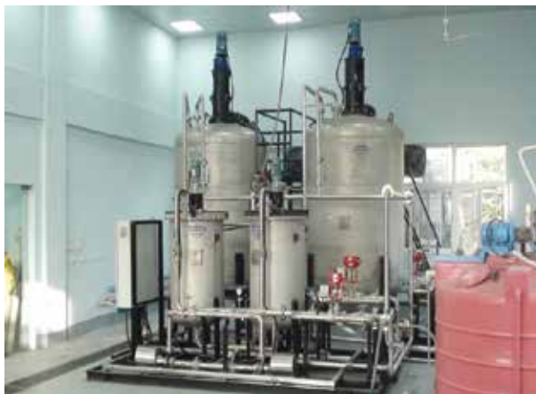
Contaminated Water Simulation Facility
