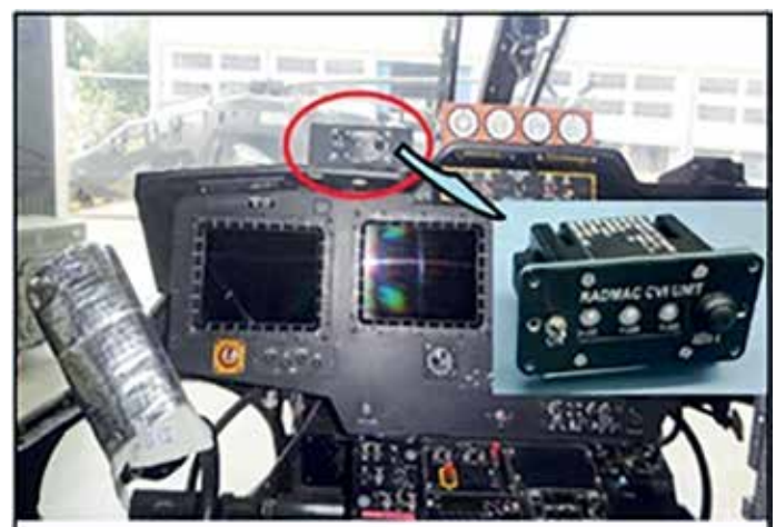
CVI Installed on Cockpit of Helicopter
