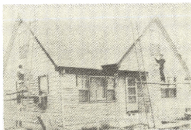
Fig. 29 Cladding external walls with terox imitation stone facing made from glass-polyester panels
